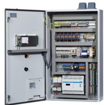
DDC cabinet for open- and closed-loop control
